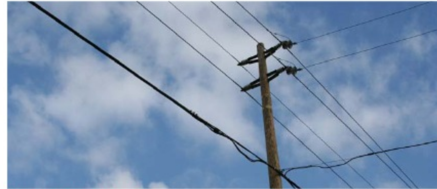
EXISTING TRANSMISSION LINE
